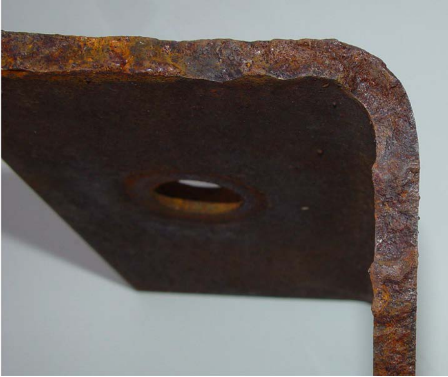
Figure 2 Lifter showing the cracked lugs. These lugs had been welded to the shell and had fractured through the HAZ of the weld.
