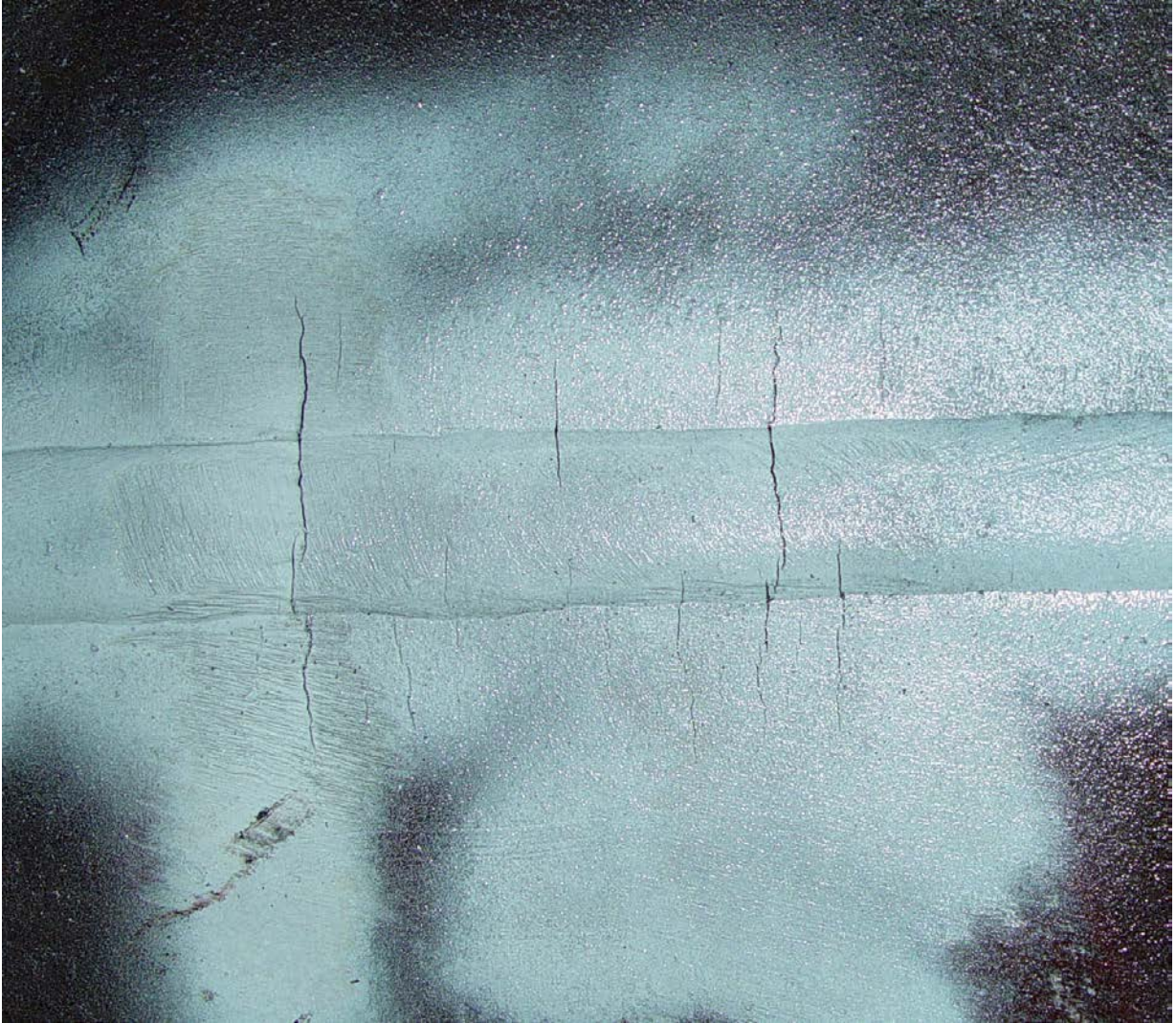
Figure 3 Transverse cracking in seam welds.
